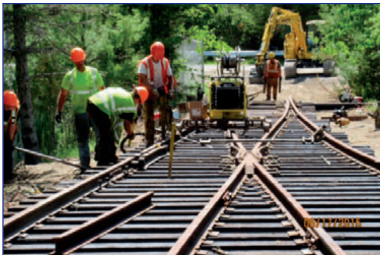
Rail lines into the site are being upgraded for the transport of site and landfill soils from the former plant which will be loaded into secured rail cars for disposal at licensed disposal facilities off site
